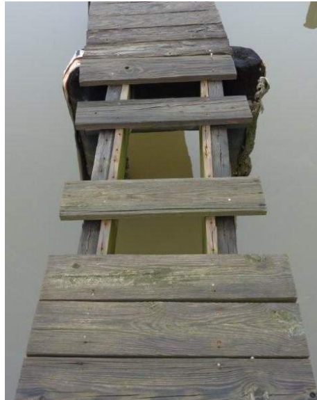
Loose and missing boards are just part of the safety hazards present on the docks and piers.
